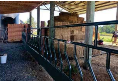
After photo of the new heavy use area. Photo by Matt Claussen
