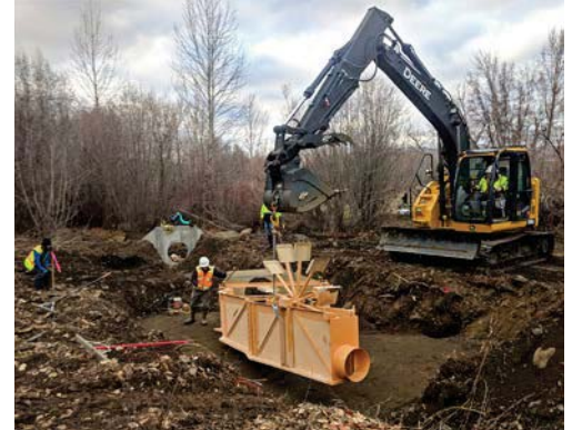
Constructing the rotary drum fish screen that will prevent fish from becoming stranded in irrigation diversion ditches. Photo by Michael Tobin
