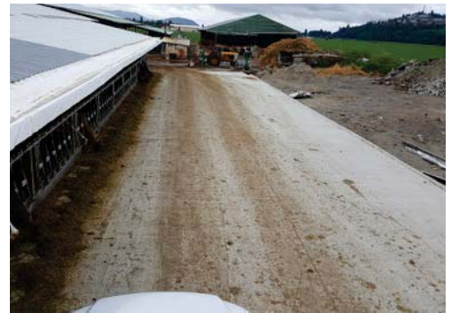
New slab and roof runoff diversion system
