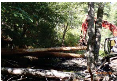
Building a logjam for salmon and steelhead habitat on Rattlesnake Creek. Photo by Dan Richardson
