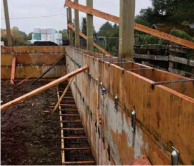
Forming the walls of a dry stack wall on a structure used to safely store livestock manure. Photo by Nikki Atkins
