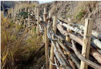
As a foundation for sediment deposits, woody debris is installed behind this bank stabilization project. Photo by Emily Novack
