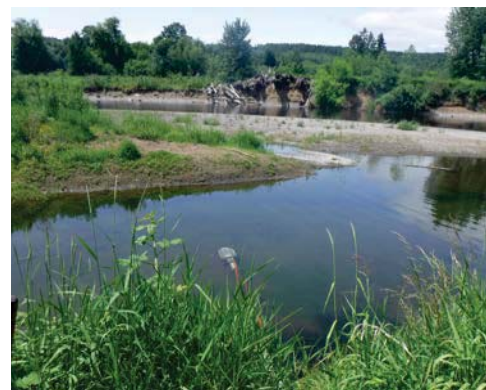
Newly installed fish screen in the Chehalis River. Photo by Kelly Verd
