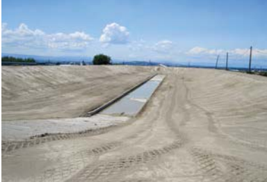
A newly constructed dairy settling basin with a concrete slab for easier clean-out. Manure solids are separated and composted.
