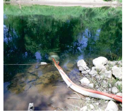
Newly installed fish screen in the South Fork Chehalis River. Photo by Kelly Verd
