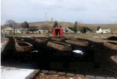
Awarded a National Association of Conservation Districts (NACD) Urban Ag Grant for new Endicott Community Garden. Construction of site is currently underway. Photo by Andrew Wolfe
