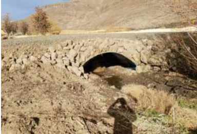
Open bottomed culvert on Meadow Creek to remove high sediment with the need to cross the creek all year round. Photo by Duane Bartels
