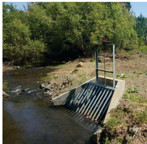
Finished headgate and fish screen installed at point of diversion. Photo by Justin Bader
