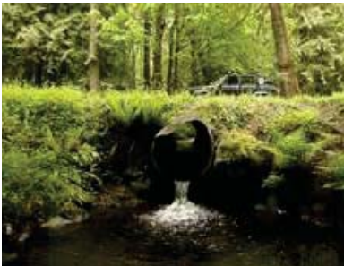
Sponsored two Family Forest Fish Passage Projects that replaced fish barriers, such as this culvert, with bridges.
