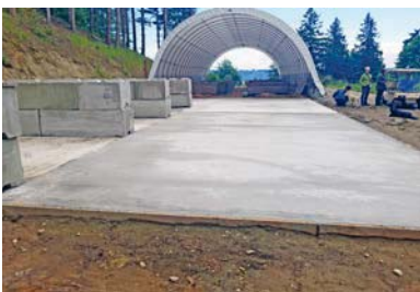
After: Cost-shared BMPs include installing a livestock waste storage facility and heavy use area protection.
