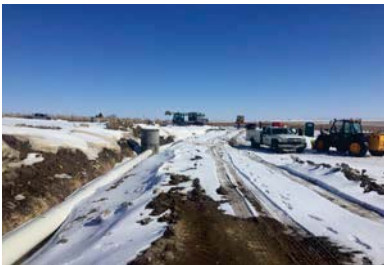
Partnered with Quincy Irrigation District and local landowner to bury an irrigation ditch in pasture preventing contamination and bank erosion. Photo by L. Stoltman
