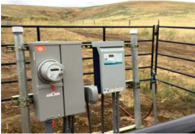
Electrical for livestock watering facility on Deadman Creek. A well was drilled and pipeline installed to move livestock from the stream. Photo by Duane Bartels
