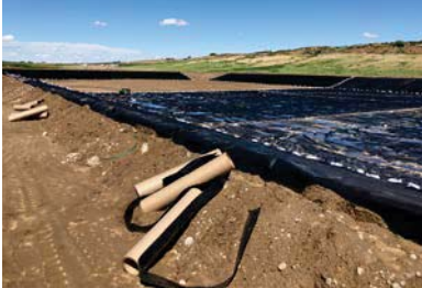
Installation of another lined dairy lagoon near the Adams-Grant County line. Photo by L. Stoltman
